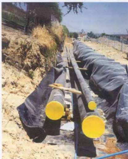
Laying the first 600m of transfer line from the fuel tanks to the outer fence at Madrid airport
