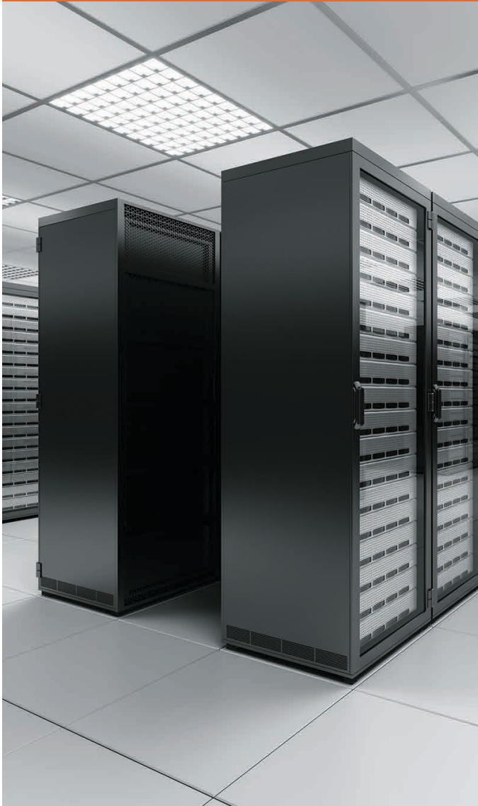
Data Centre & Comms Rooms
