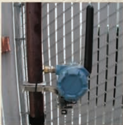
Mesh Wireless Link to the Control Room
